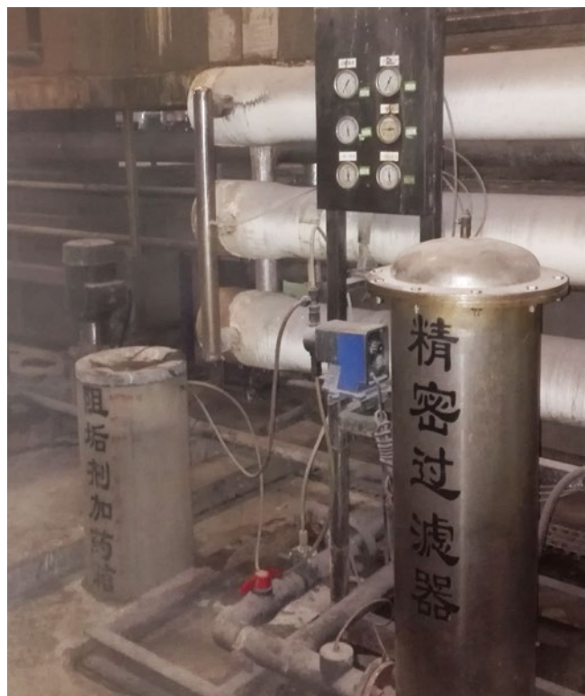
Installation traitant l'eau pure.
